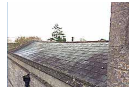
Etton, St Stephen, damaged Chancel roof in 2018
