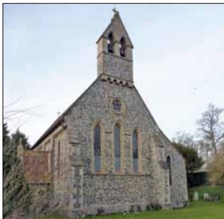
• The RC church of Our Lady Immaculate and St Philip Neri at Kirtling received a £2000 grant for the repair and protection of the west window glazing.
