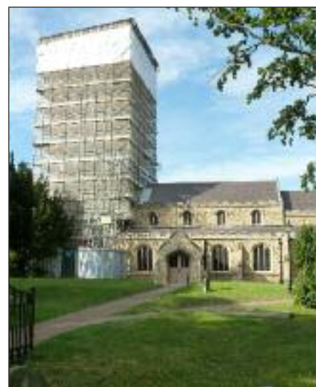
• Littleport, St George: The Trust's £3000 grant and £15,000 loan might seem a small contribution to this £250,000+ tower repair, but it was a third of the shortfall required by the parish to match the English Heritage grant.
